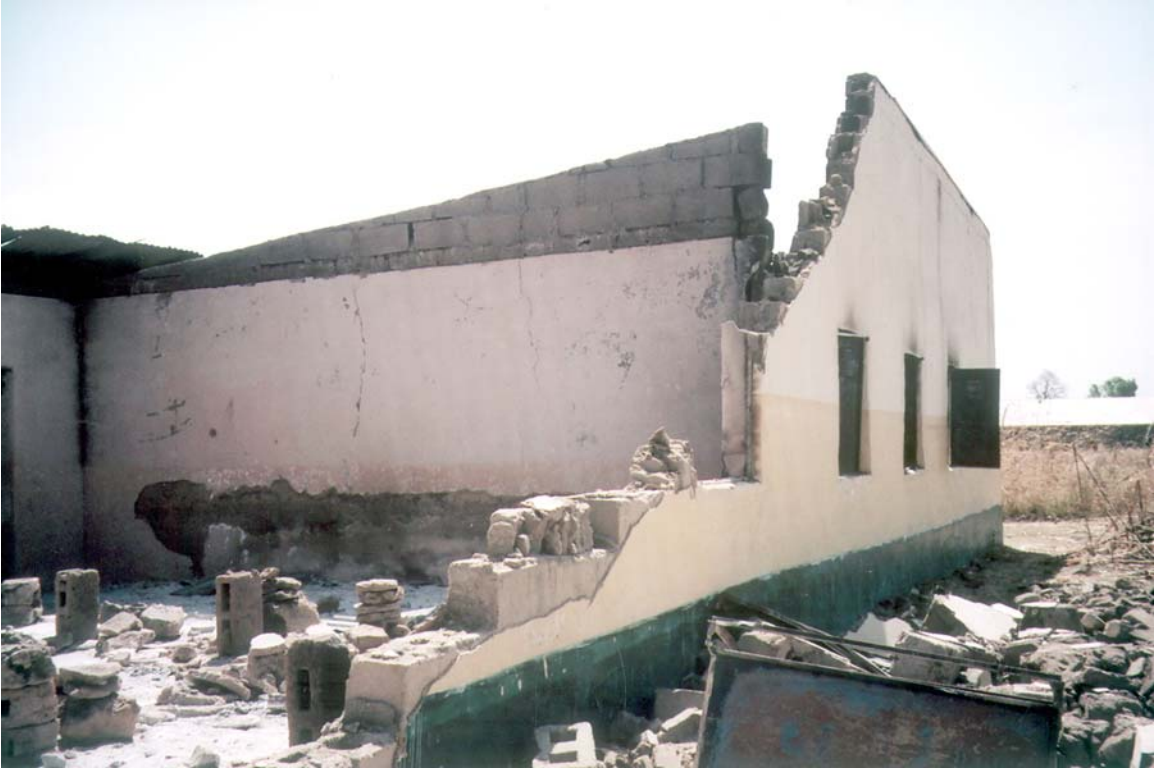
Primary school in Nariya, destroyed in November 2002. © 2002 Human Rights Watch
